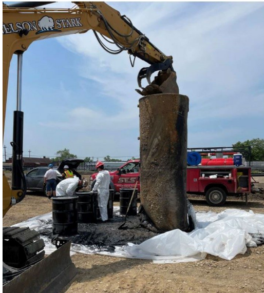
(ABOVE) The Butler County Land Bank was able to grant the City of Hamilton funds for the removal of abandoned gas tanks at the site of the city's new Justice Center. This allowed the project to stay on budget and on time.
